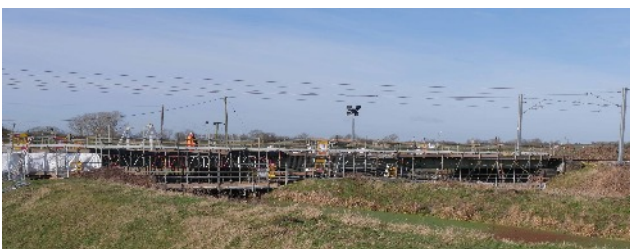
Work on the Great Catchwater Drain viaduct caused the blockade. Photo: Steve Smithson
